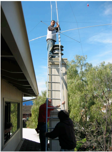
George views at the window with safety in mind. Roofer is 40 ft. up!!
